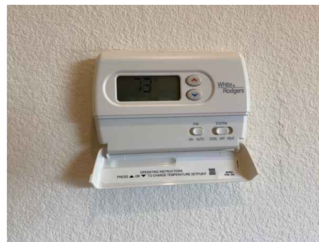
Thermostat Controls: Thermostat
